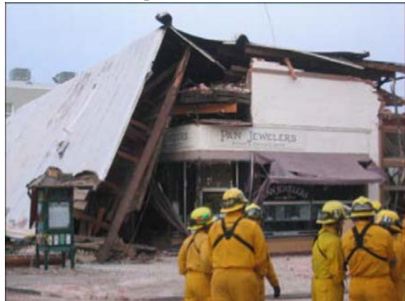
The Acorn building in Paso Robles collapsed in the December 22, 2003 San Simeon earthquake, killing two people. The building was torn down within weeks so data for an engineering analysis of why it collapsed had to be collected quickly.
