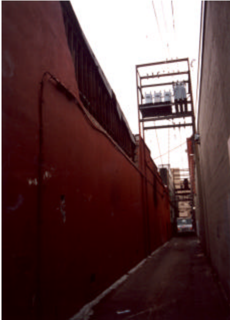
Figure 1. Platform Mounted Transformers, Olympia, WA
