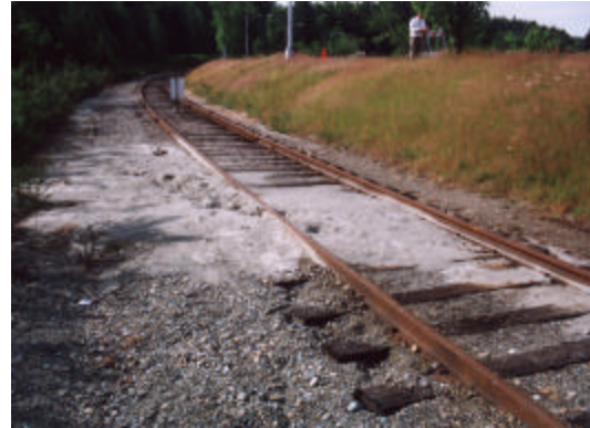
Figure 2 Sand Boil at Rail Road Track, Deschutes Parkway, Olympia, WA
