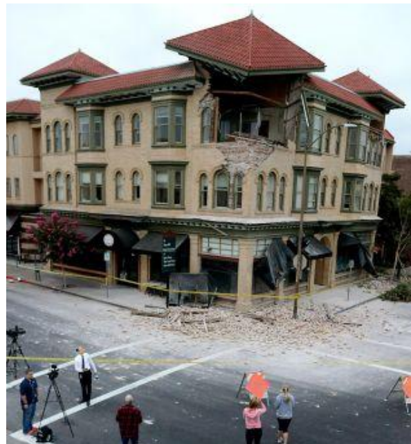
Collapse of the Alexandria Building after the 2014 South Napa earthquake.
